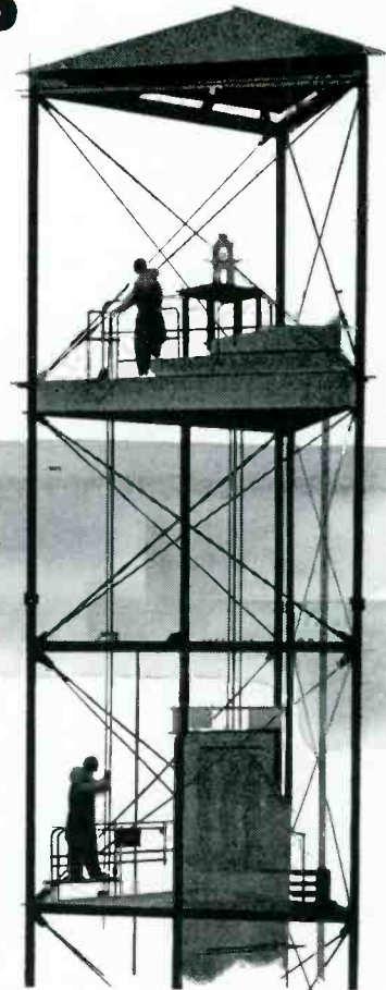
Long elevator ride takes men up to within 24 feet of top. They mount ladder for final ascent.
